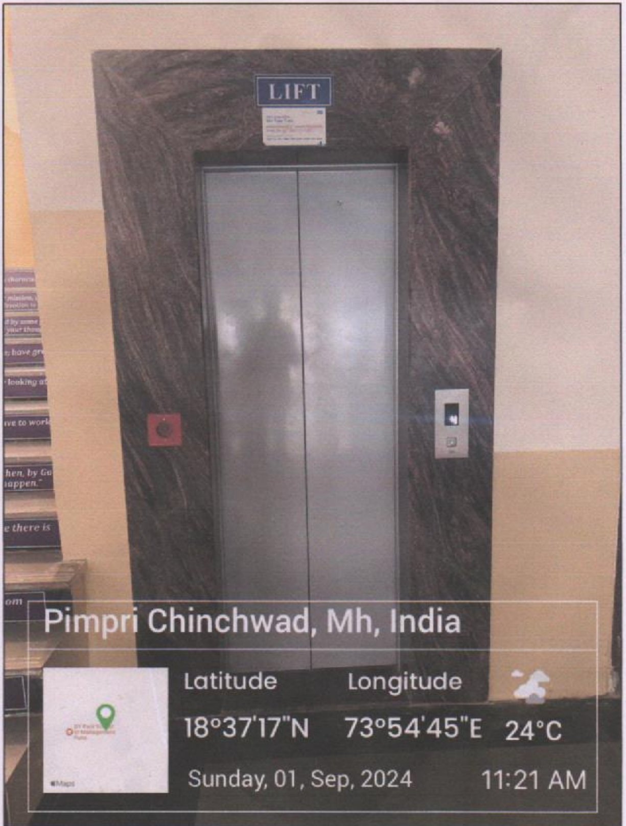
Lift at DYPSOM building
