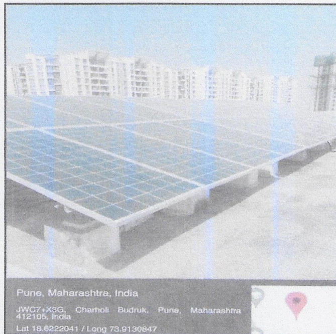
Photograph of Roof Top Solar PV Plant:
