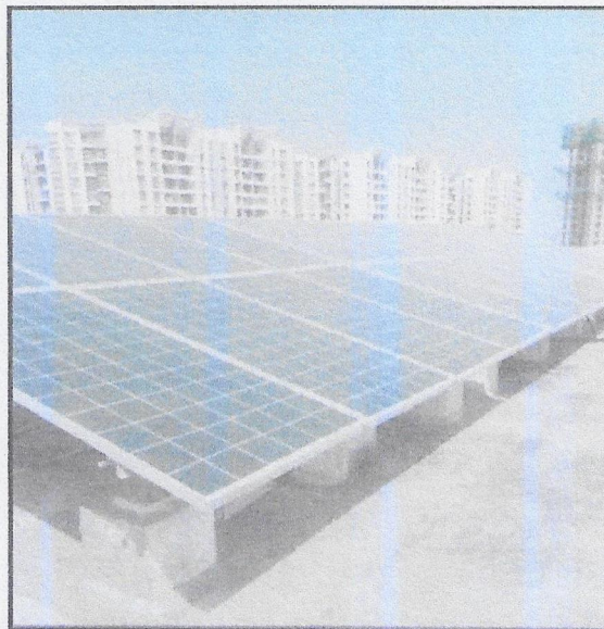
Photograph of Roof Top Solar PV Plant:
