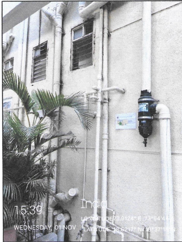
Rainwater Harvesting at campus
